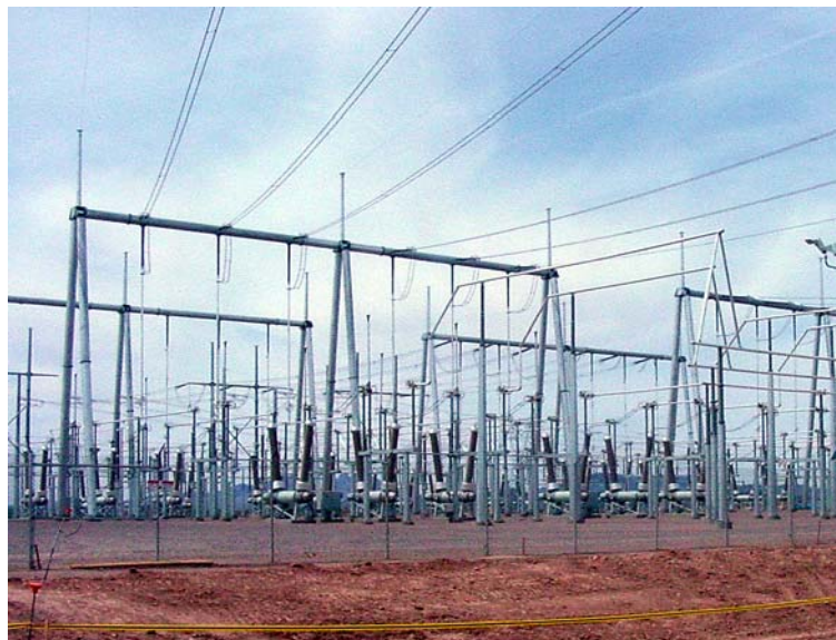
Switchyard & 500 kV Line Exits
