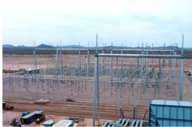
Switchyard Viewed from Plant Site
