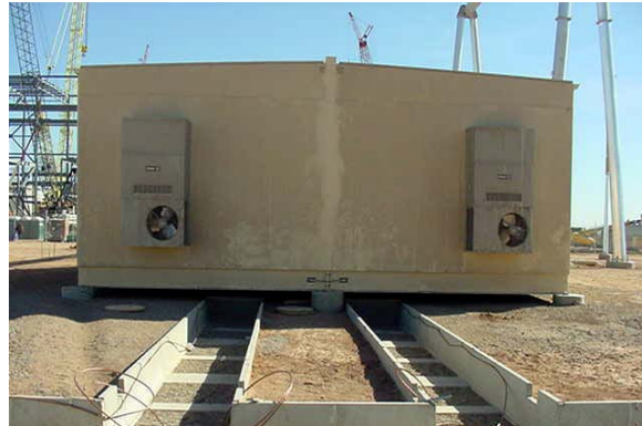
MODULAR CONTROL BUILDING
