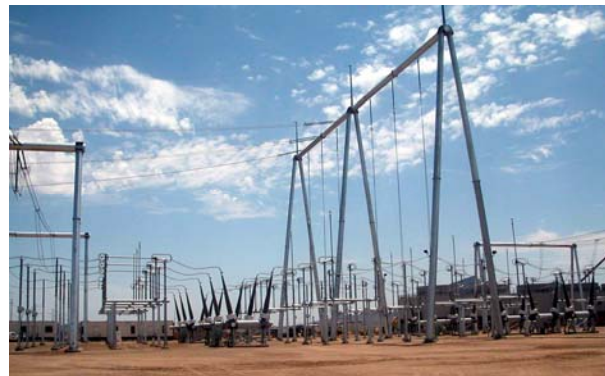
500 kV Yard Area
