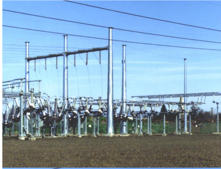
E.E. Clouse Substation
