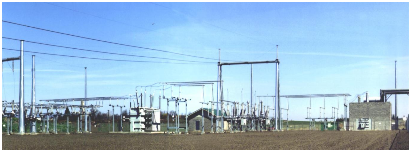
E.E. Clouse Substation
