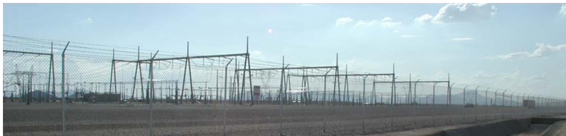
Profile of 500 kV Strain Bus Towers
