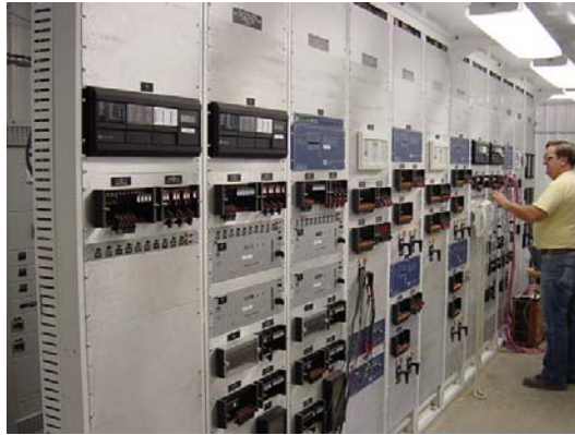
Extensive Relays & Controls
