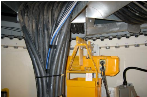
Tower Internal Wiring
