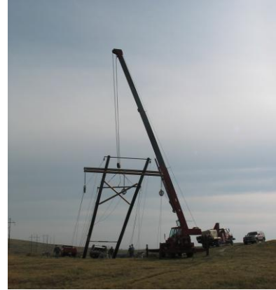
Pennel Transmission Line
