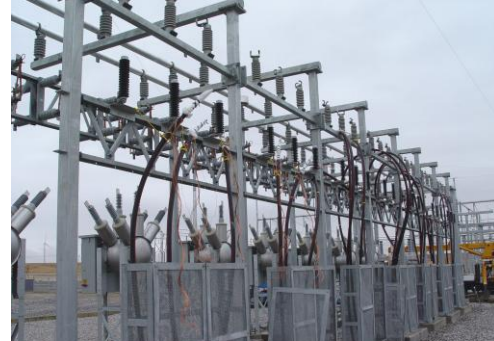
Judith Gap Substation
