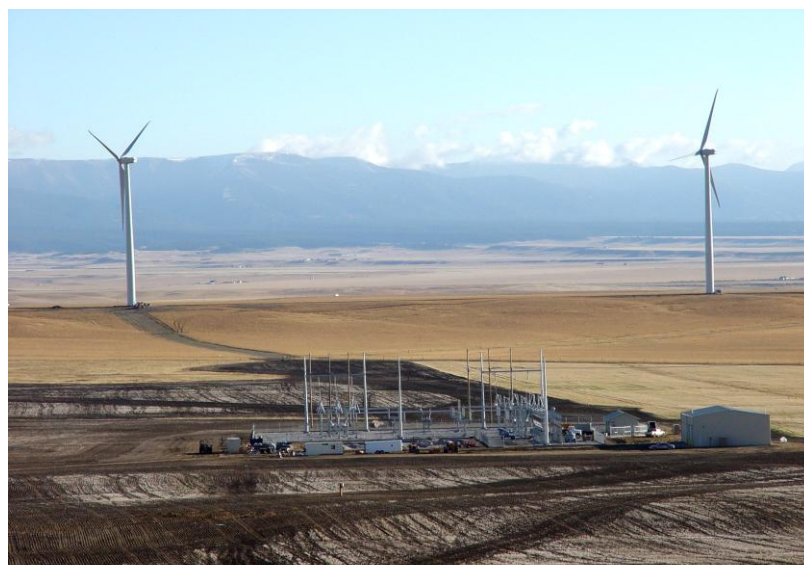
Judith Gap Substation
