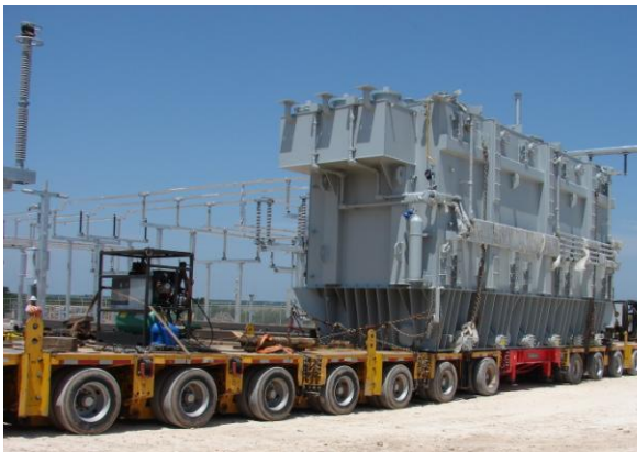
345 kV – 555 MVA Transformer
