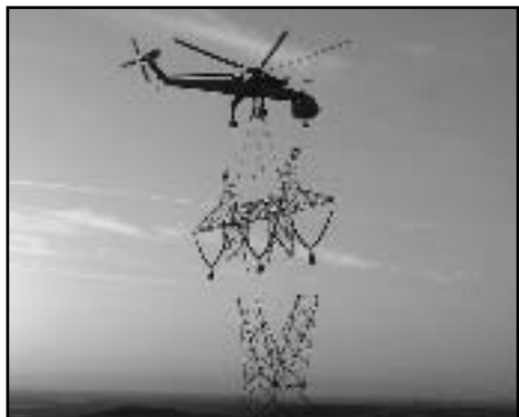
A total of 245 lattice steel towers were built for the Path 15 project.
